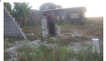
Fallen Remand Home perimeter wall - Bo
